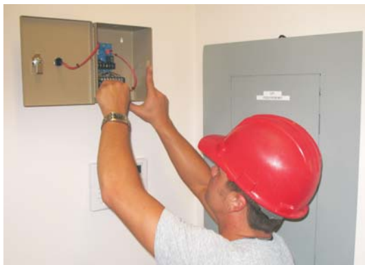
Dedicated terminals on the logic panel facilitate easy wiring. Auxiliary terminals can also be wired to a central alarm system.
