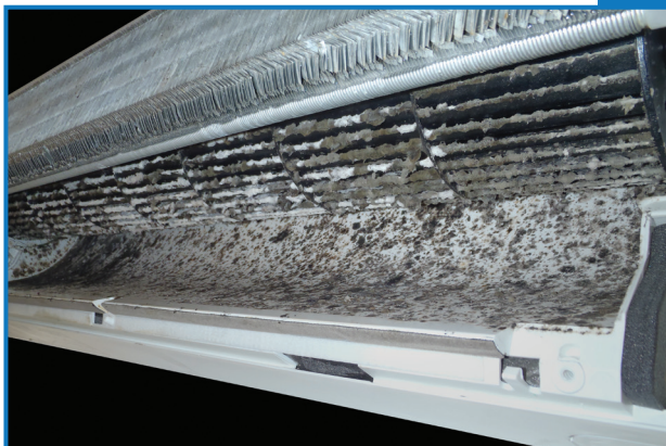
Mini-Split blower with MOLD
